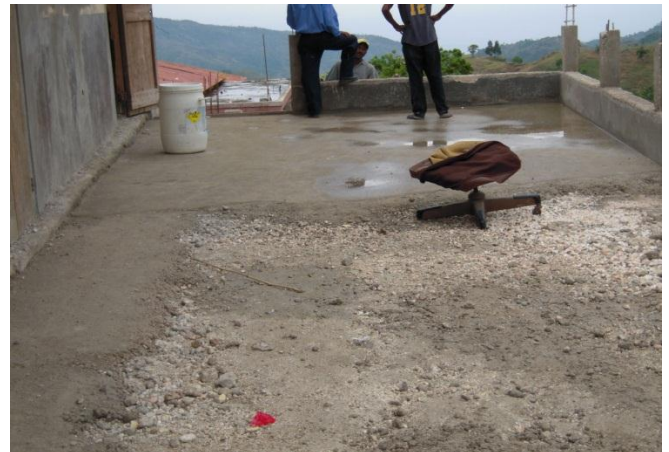
School of St. Therese in Laval, work in progress on the terrace.
