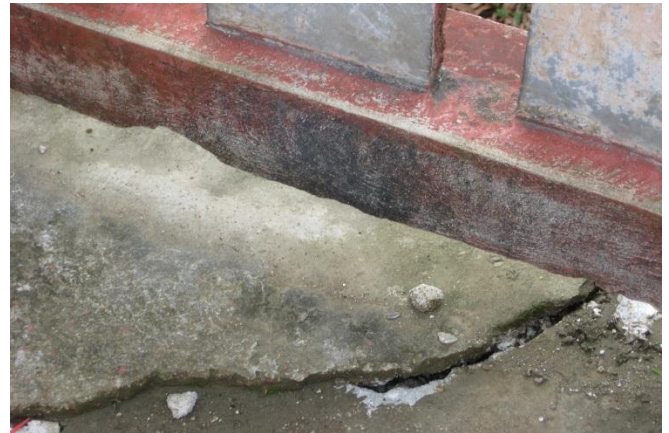
School of St Therese in Laval: Many cracks in the walls and floor. Terrace and doors are also damaged and need to be rebuilt. The building is solid.
